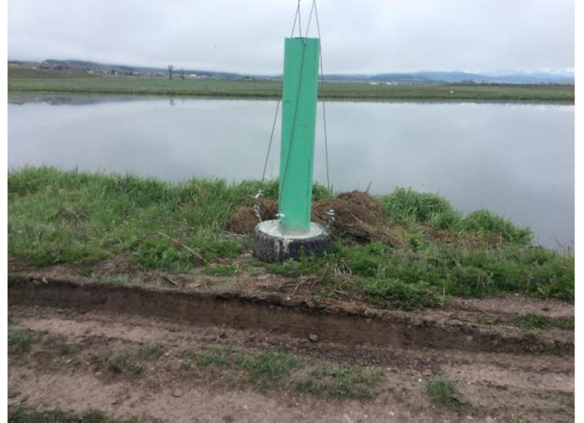
Picture 6. Leak Test Pipes Installed Using Lift Hooks in Cell 1 on May 23, 2018
